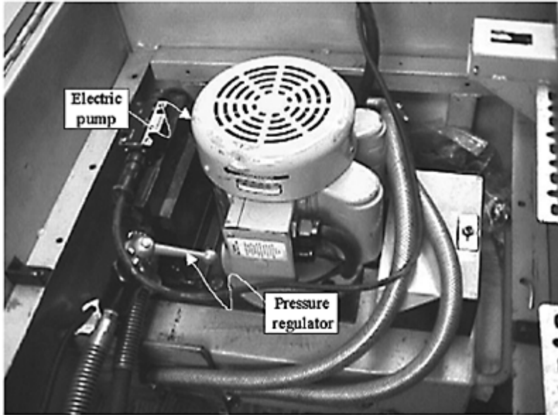
Figure 9.15 Electrical pump used to supply fluid to hydraulic jacks.
