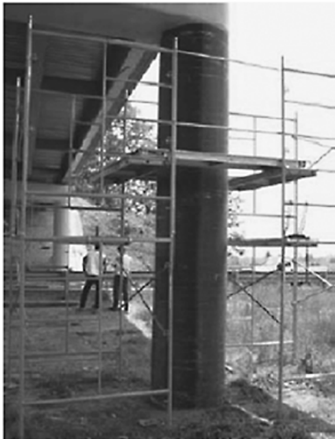
Figure 1.3 Column wrapping with carbon tape, followed by coating of inorganic resin (a) column after cleaning; (b) column wrapped with carbon tape; (c) during final coating application; (d) column after coating (Source: Defazio et al. , 2006).
