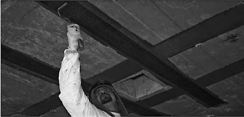
Figure 1.2 Hand lay-up process used to strengthen reinforced concrete slab (Source: Structural Preservation Systems, 2007).
