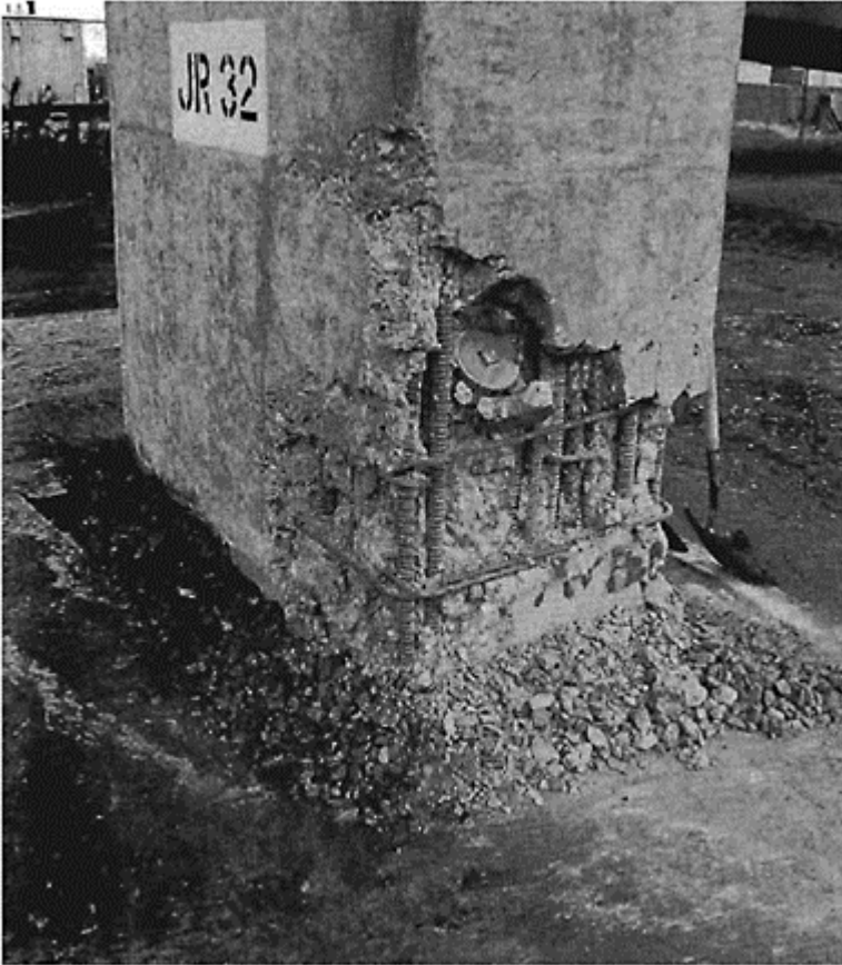
Figure 8.13 Lap splice bond failure during Loma Prieta Earthquake, 1989 (Source: Priestley, M. J. N., Seible, F. and Calvi, G. M., Seismic Design and Retrofit of Bridges , © 1996 and owner. Reproduced with permission of John Wiley & Sons, Inc.).
